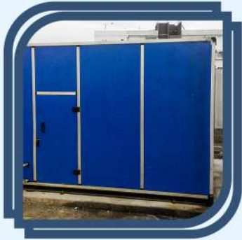
Fresh Air System
