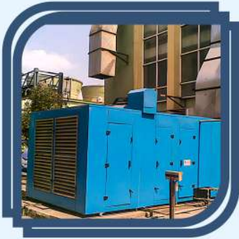
Pressurization & Ventilation System
